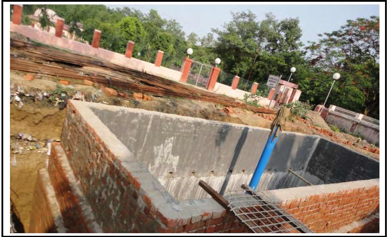
Fig. 11.1: Construction of Recharge Pit near New Petroleum Engg. Building, ISM campus Dhanbad (Side View)
