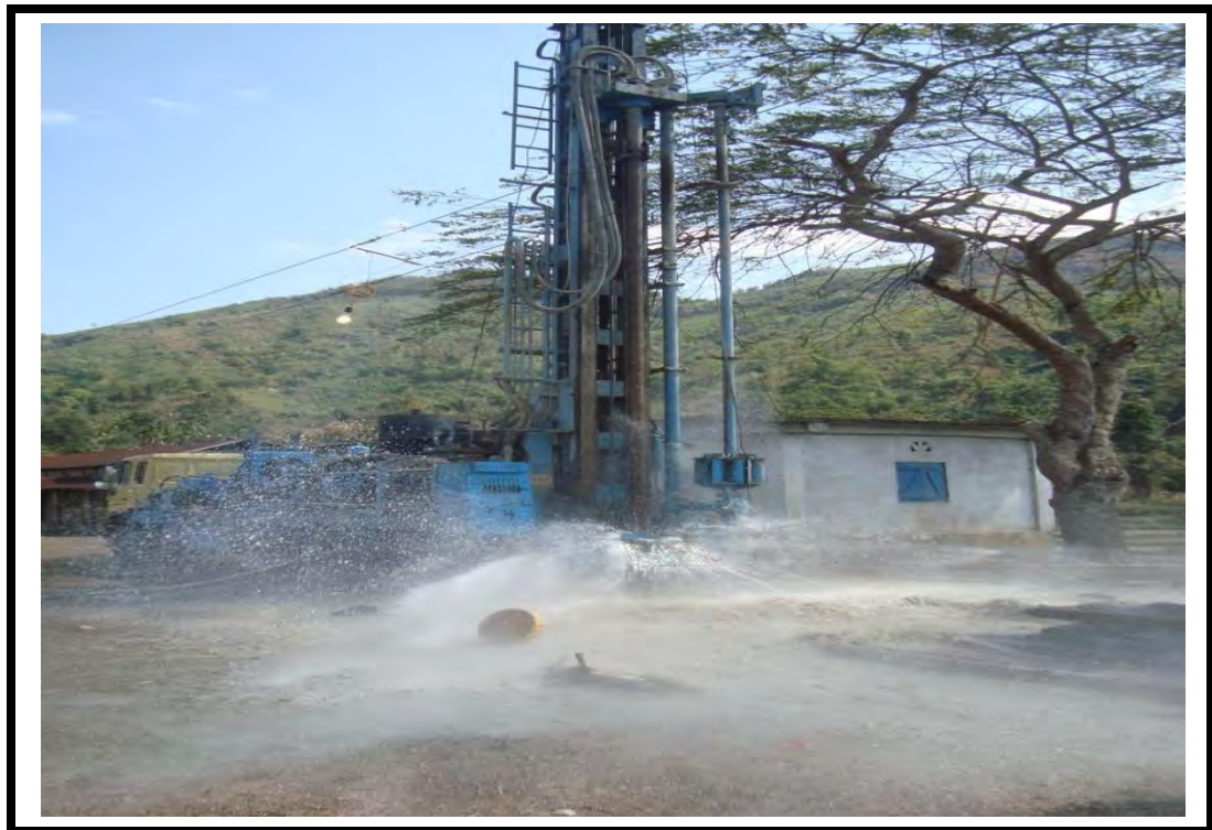
Fig 4.8 High Discharge Exploratory Bore Hole at Nongladew Village, Zirang Block, Ri-Bhoi District, Meghalaya
