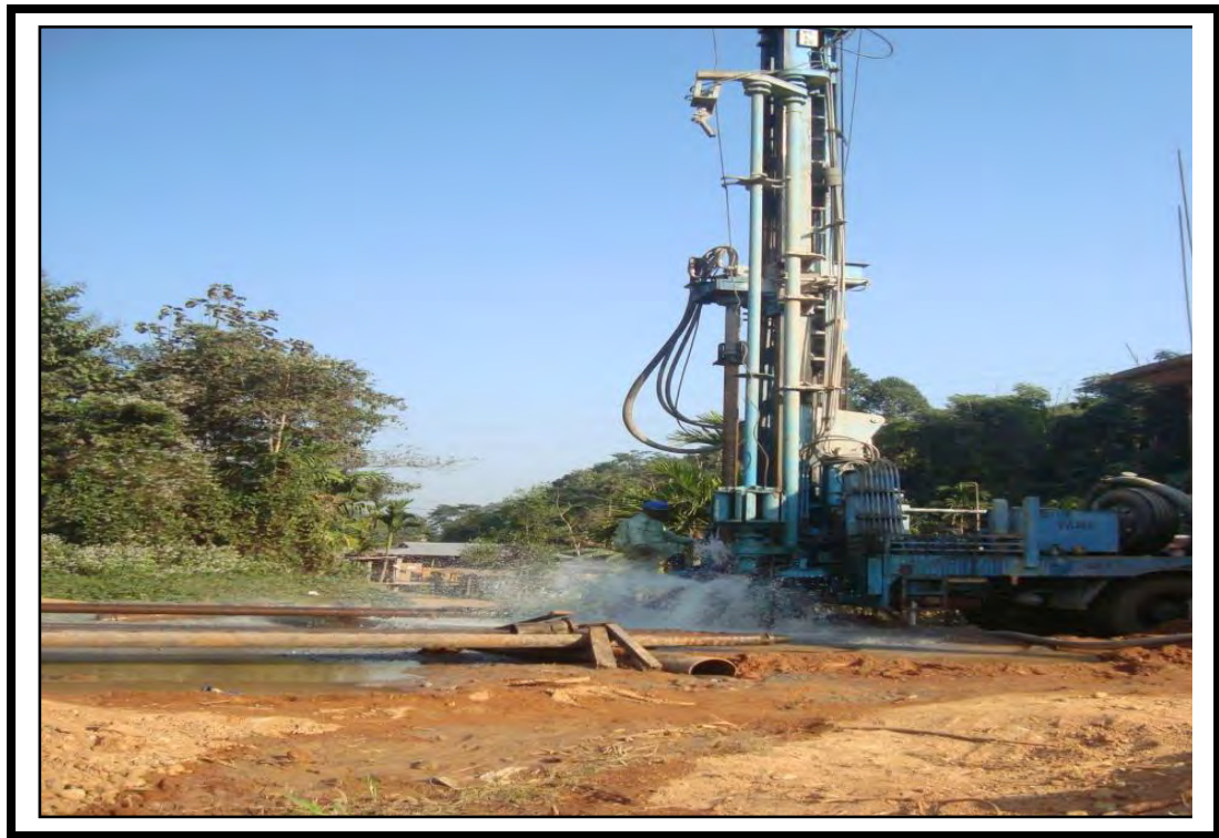
Fig 4.7 High Discharge Exploratory Bore Hole at Umling Village, Umling Block, Ri-Bhoi District, Meghalaya
